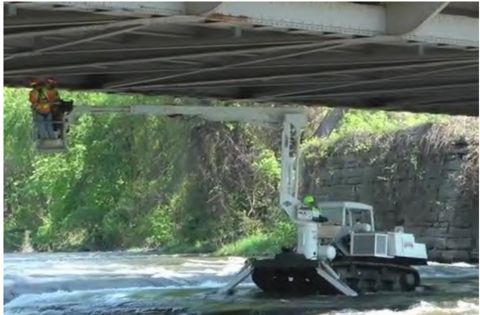
Figure 2.5.18 Track-mounted Man-lift in a Stream
